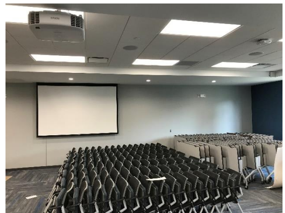
Projector and projector screen installed in Multi-Purpose Room
